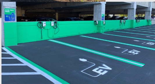
EV charging, Madisonville Operations Center, Cincinnati, OH
