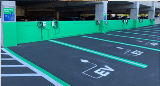
EV charging, Madisonville Operations Center, Cincinnati, OH
