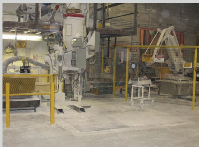
New bagging machine and south robot
