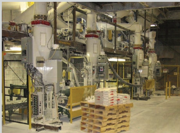
Four of six new bagging machines with south robot in the background
