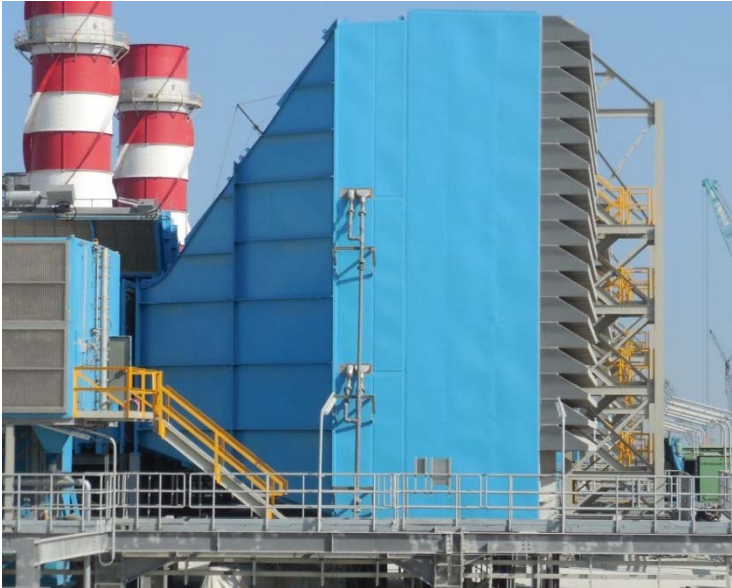
Gas turbine filters
