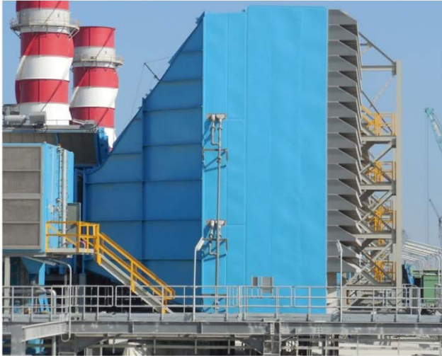
Gas turbine filters
