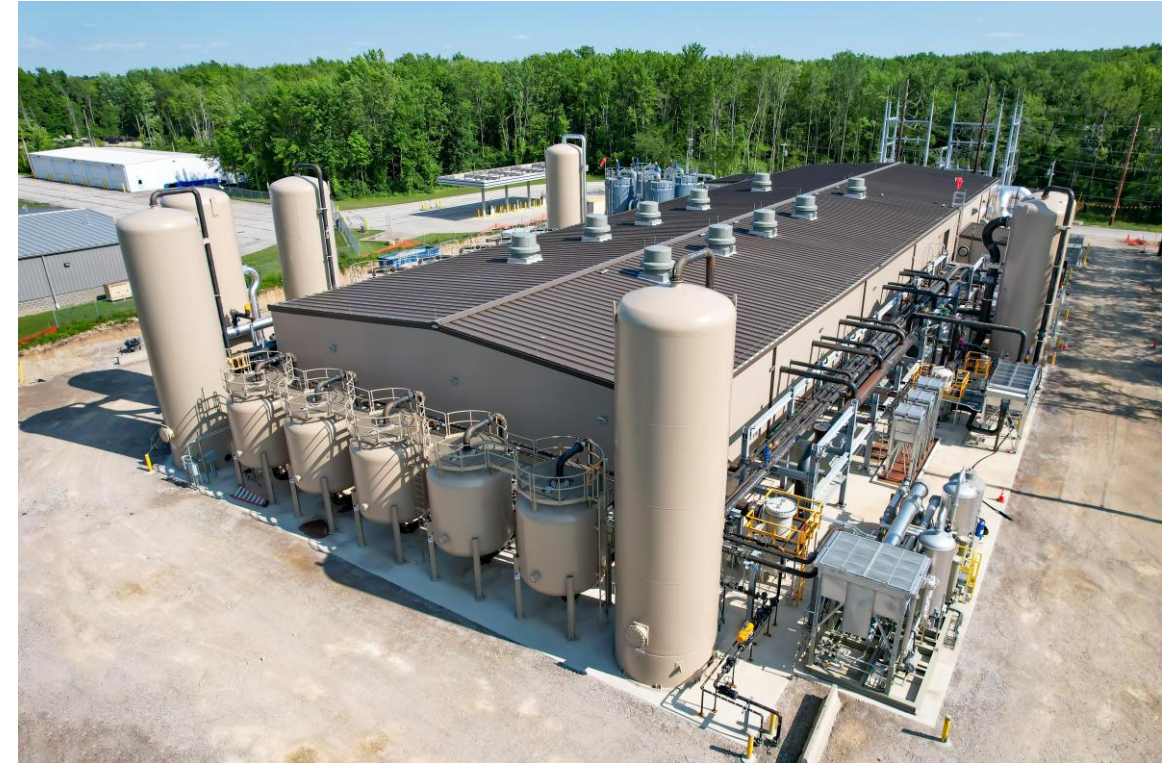
Lorain RNG Facility, one of two projects with EDL
