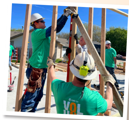
In Norman , more than 40 Oklahoma Natural Gas volunteers from Operation teams across the Oklahoma City area cut lumber and constructed and erected the home's exterior walls.
