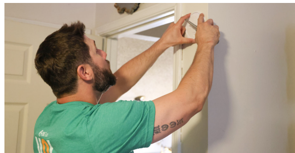
Volunteers install smoke detectors at the American Red Cross Sound the Alarm event in Tulsa.
