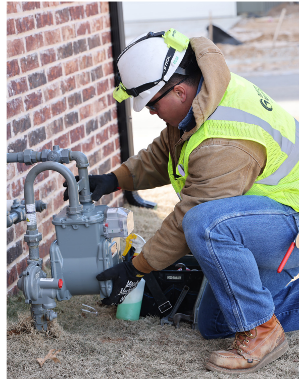
A service technician connects a gas meter.
