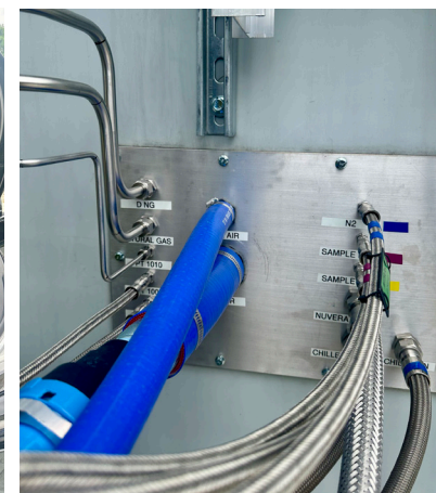
Methane reformation equipment, which generates hydrogen from renewable natural gas sourced from a Texas landfill and supplied by Texas Gas Service.
