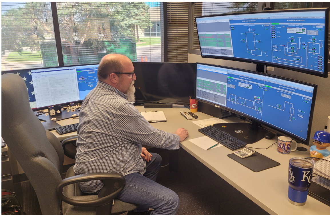
Gas Control is staffed around the clock for reliable and safe delivery of natural gas to ONE Gas customers.
